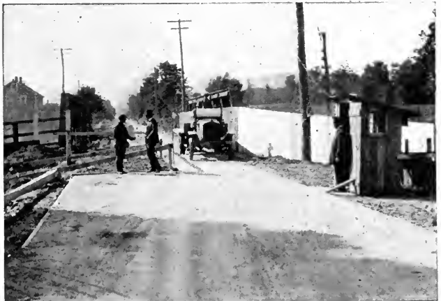
WHEN THE HALF-AT-A-TIME METHOD PERMITS ONLY ONE LINE OF TRAFFIC, THIS IS REGULATED BY A TELEPHONE, IN MASSACHUSETTS
